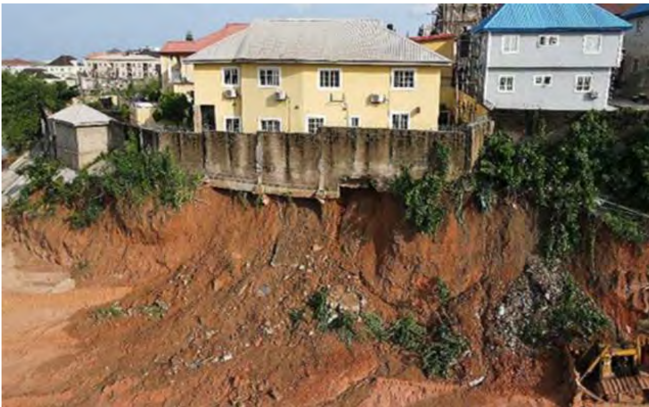
Effects of erosion on some houses
